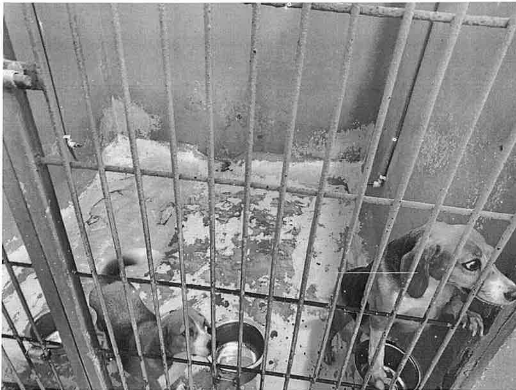
Photo 9: Stained and poorly maintained flooring
